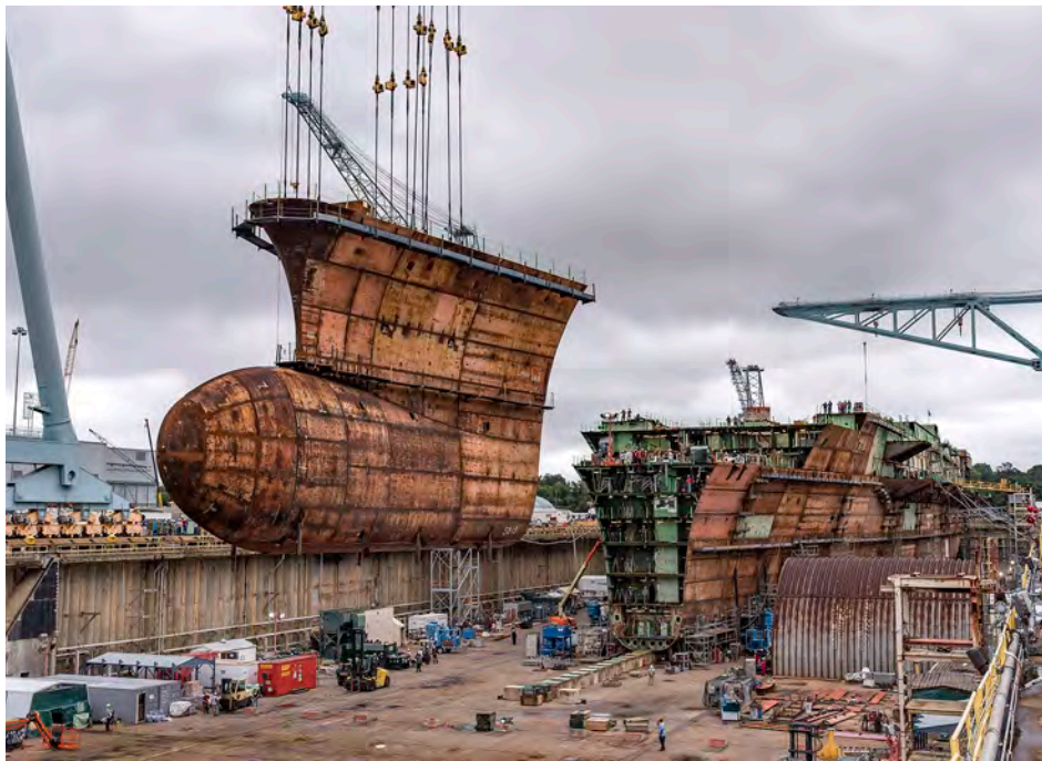
CVN 79 Lower Bow Positioned in Dry Dock. Courtesy of Huntington Ingalls Industries - Newport News Shipbuilding.
